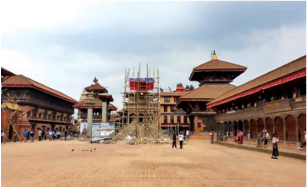
Figure 1 Reconstruction works going on in Bhaktapur Durbar Square. Picture taken:- June 10th 2019
