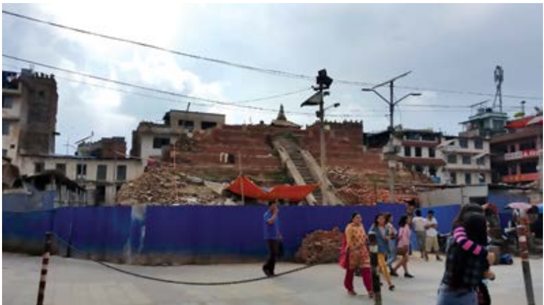
Figure 2 Reconstruction works of monument Maju Dega yet to commence in Basantapur Durbar, Kathmandu. Picture taken:- June 9th 2019
